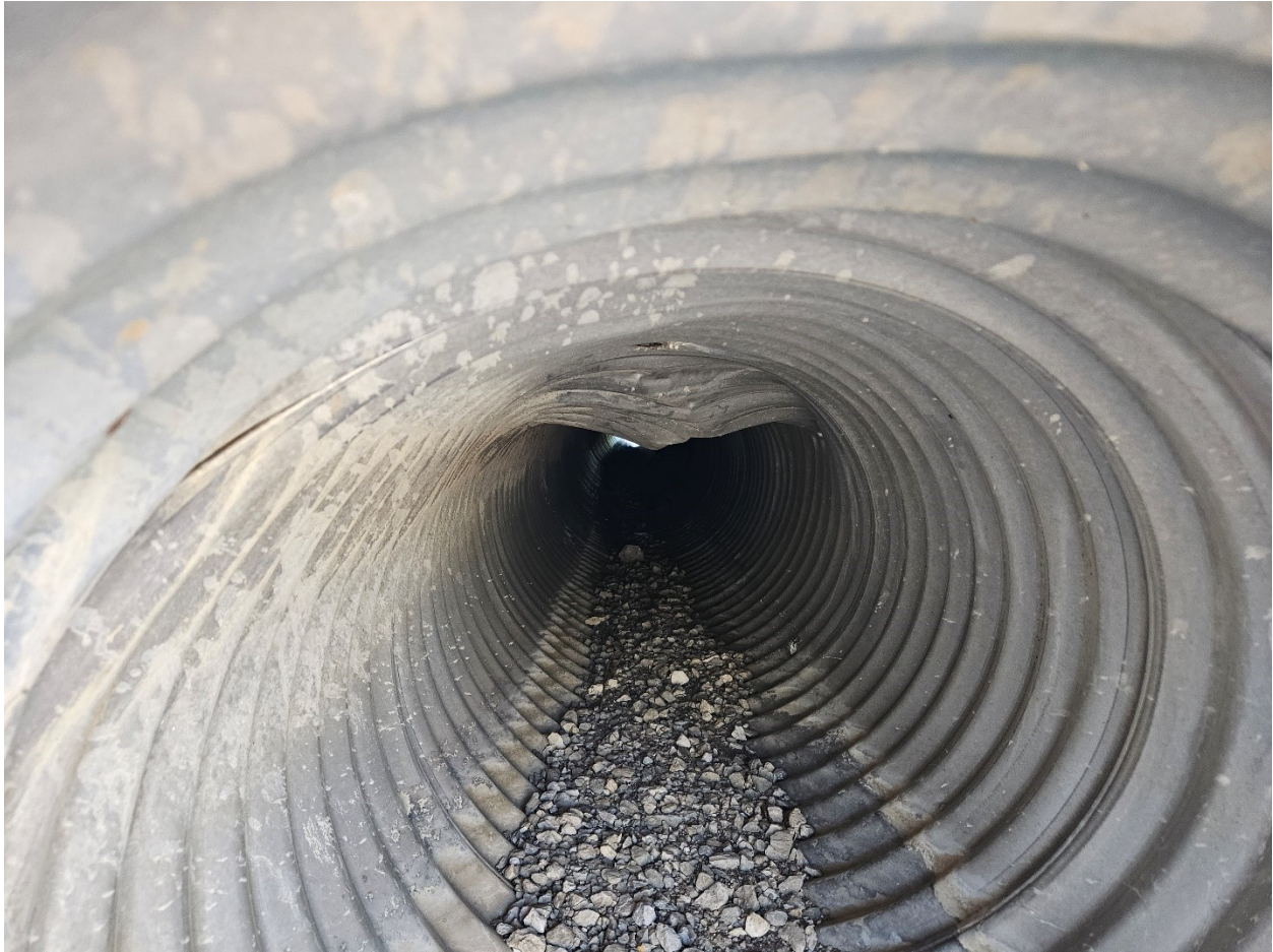
Figure 1: Crushed 24" CMP Crossroad Culvert on Stillwell Road, east of 178th Street
