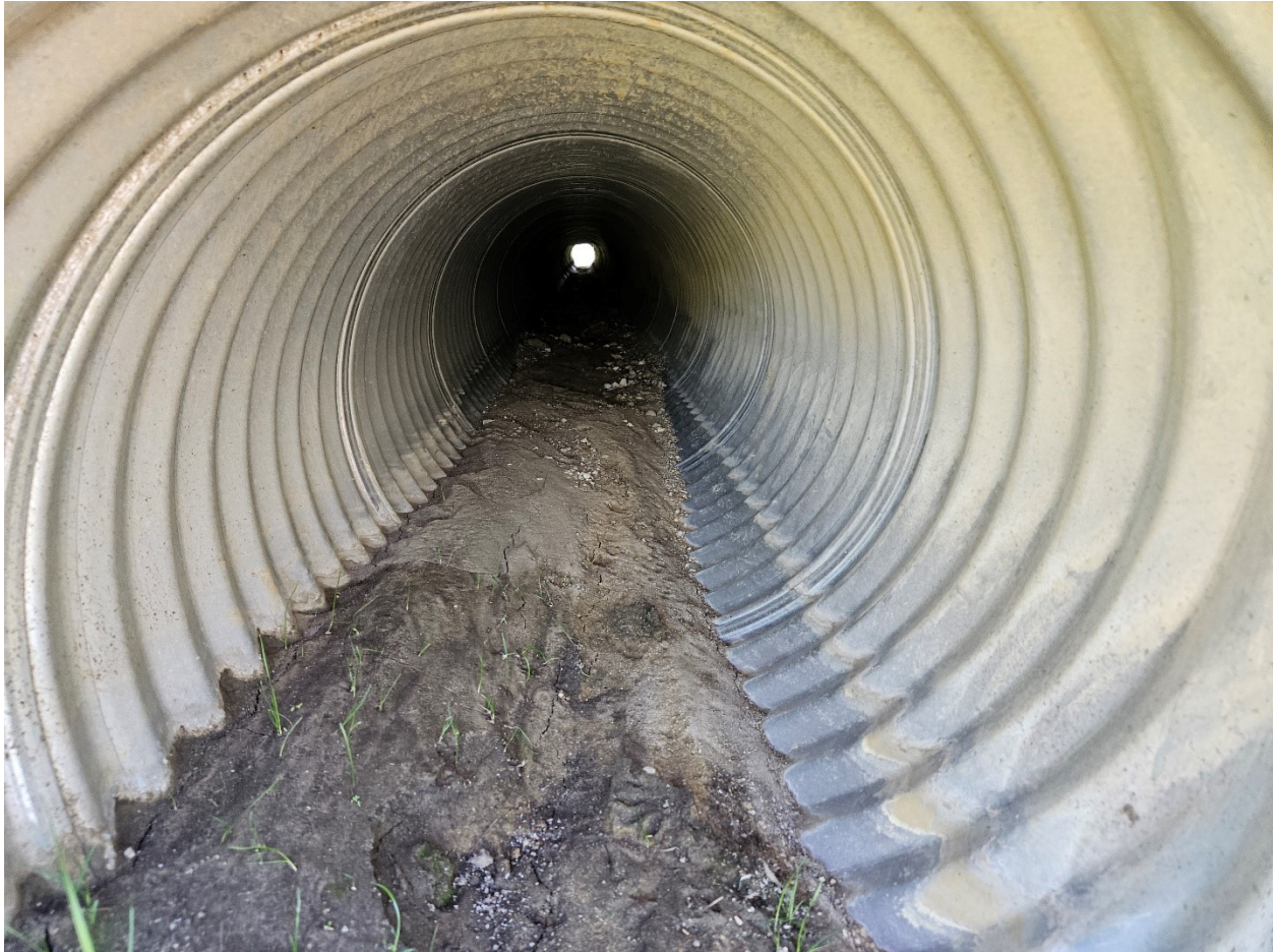
Figure 2: 24" CMP Crossroad Culvert at the intersection of K-32 Highway and Stillwell Road
