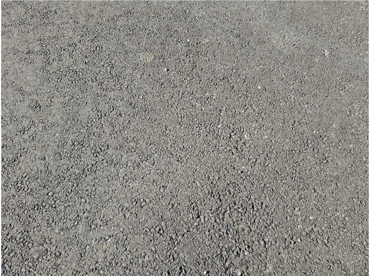
Figure 3: Asphalt Surface Segregation Example near Stillwell Road and 178th Street Intersection
